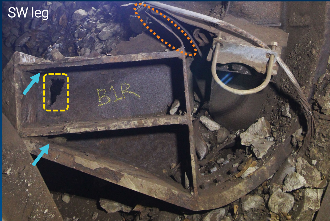
Corrosion product build-up
