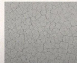
ALKALI-SILICA REACTION (ASR) CRACKS
