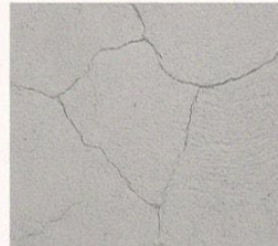
PLASTIC SHRINKAGE CRACKS
